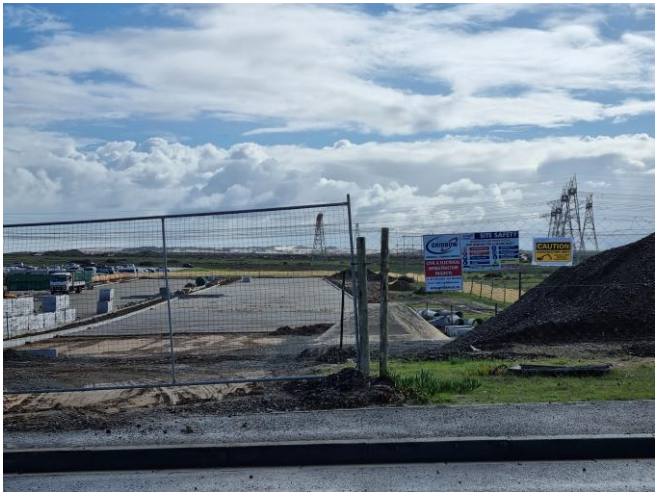
Image 11: Closed access with appropriate signage
